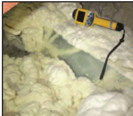
Photo 4: No foam on duct and large area of delaminating 1/2 lbs foam
