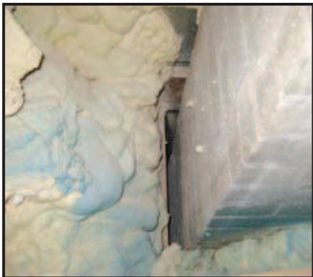
Photo 1: No seal around masonry chimney
